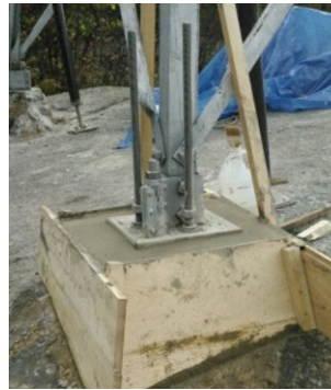
Holes drilled into bedrock, anchor bolts glued in, and concrete poured into forms.
