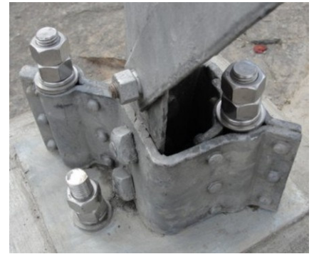
Finished job on one leg. You can see the new stainless steel bolts.
